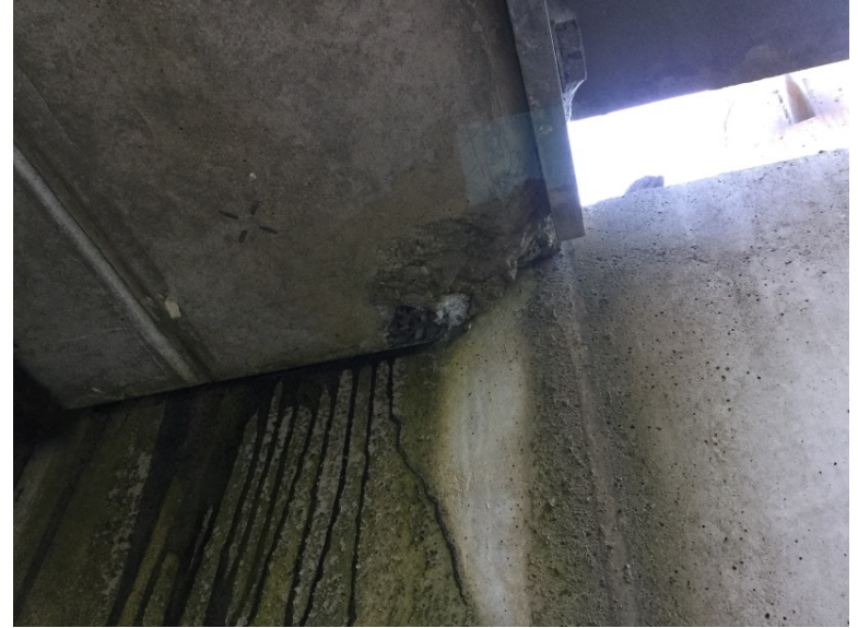
Upstream right bank deck damage
