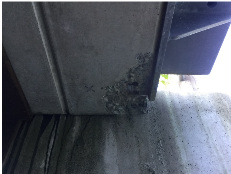
Downstream left bank deck damage
